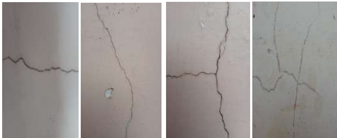
Figure-2 Sample Image of wall crack
